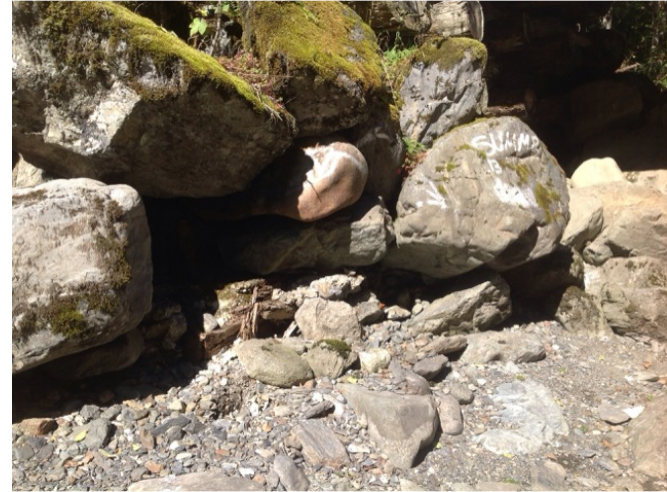
downstream right abutment scour
